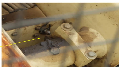
Figure 2. 500RTS 6.7 m Lift/Drive interlock limit switch location
